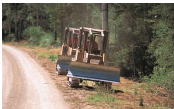
Small dozers used to clear lantana from between rows to allow access in hoop pine plantations—Yarraman, Queensland.
