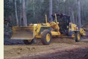
Don't move contaminated soil or fill
